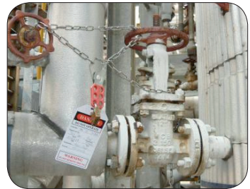
Figure 28: Example of valves and piping lockout.
