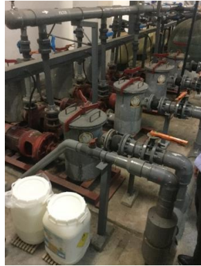
Interior of the pump room with containers of granular acid.
