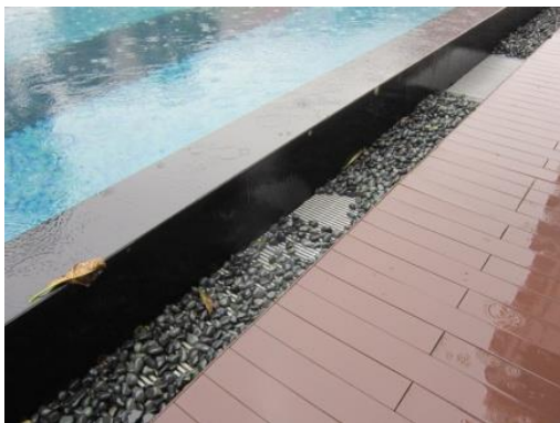
Photo of the drain where dosing was carried out.
