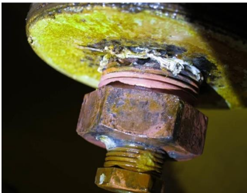
Photo of the corroded fusible plug connection
