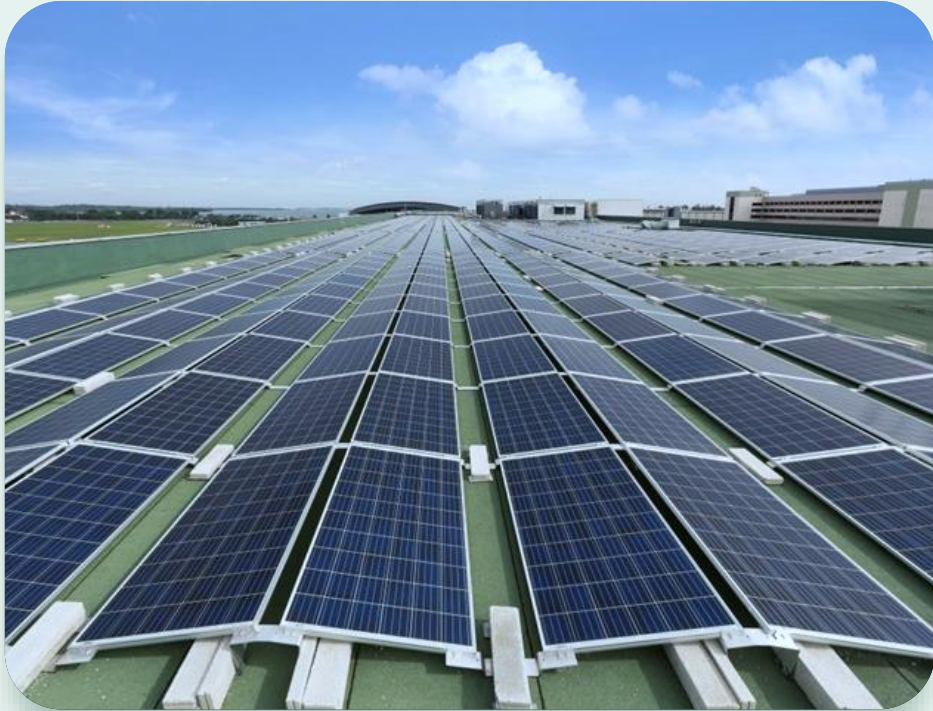
C&I Rooftop PV at Changi Airport for SATS
